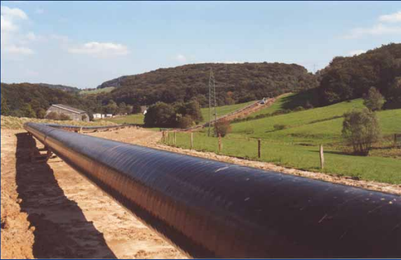
Oil and Gas Pipeline Monitoring
