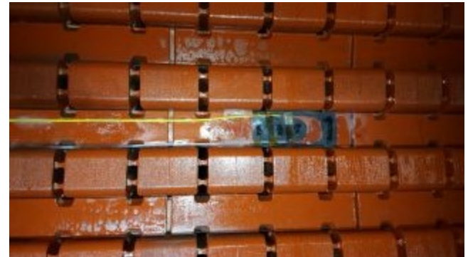
Turbine End Resin
